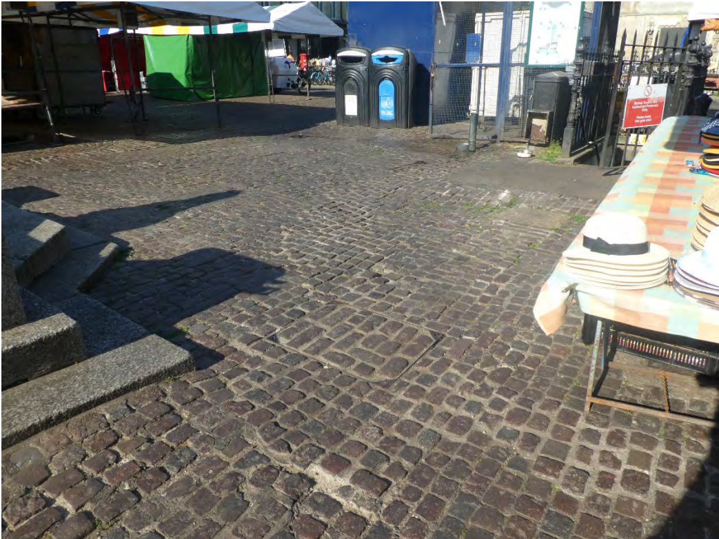
Photo 18: Zone 11 showing unevenness and worn pointing
