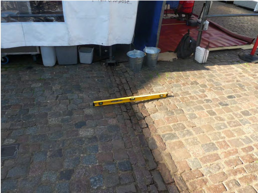
Photo 14: A 45mm deep channel on a main walkway in zone 12
