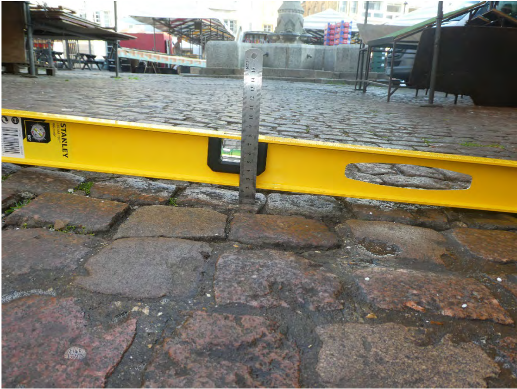
Photo 20: Undulation of 20mm on walkway in zone 3.
