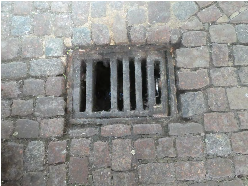
Photo 13: Broken and deeply recessed grating between zone 3 & 4.
