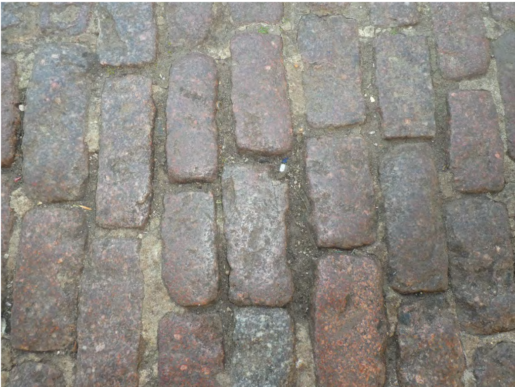
Photo 25: General view of worn pointing and rounded setts in zone 1.
