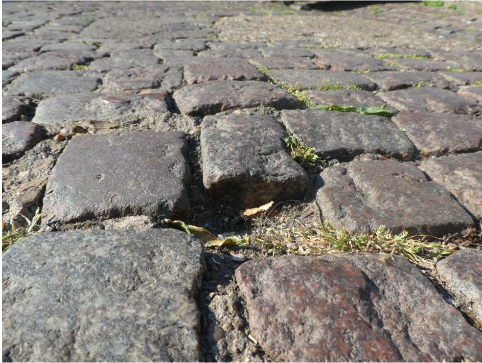
Photo 16: Significant lip, missing pointing and rounded setts in zone 11.
