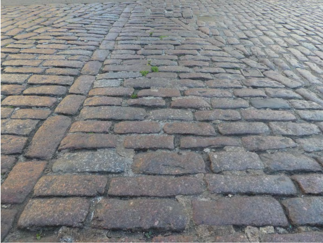
Photo 24: General view of worn pointing and rounded setts in zone 10.
