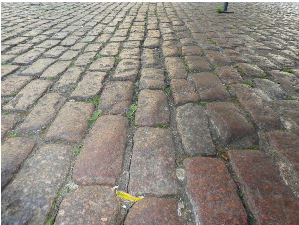
Photo 29: Zone 2 example of worn pointing and rounded/damaged setts.
