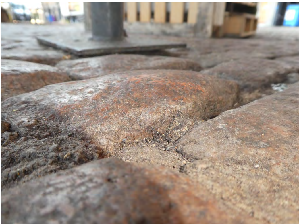
Photo 27: Example of rounded setts in zone 5.
