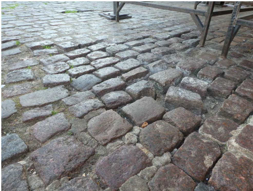
Photo 17: Loose setts missing pointing and rounded setts in zone 3.
