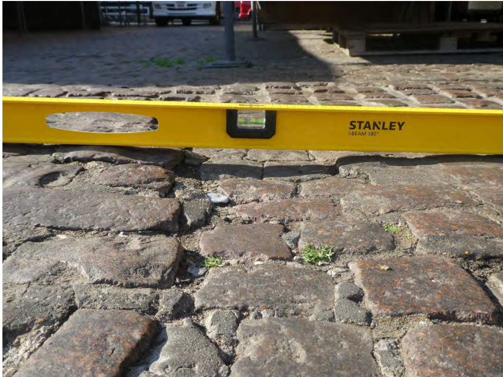
Photo 19: Zone 11 showing significant hazard and rounded/damage setts.
