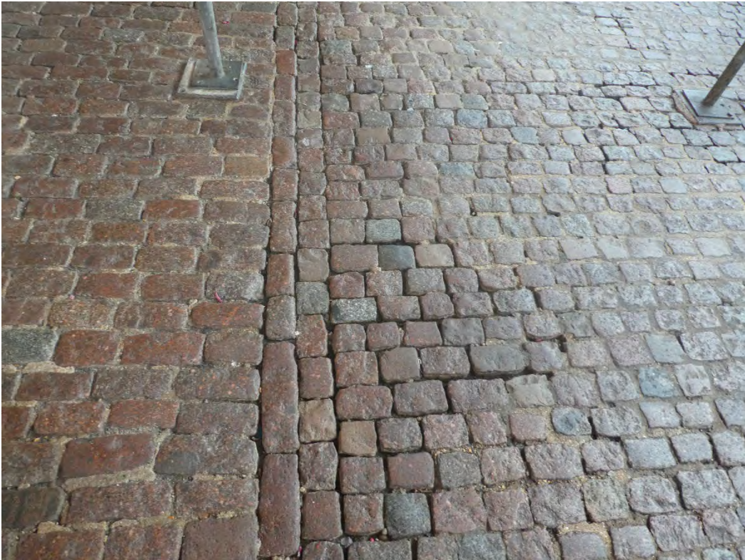
Photo 26: Missing and worn pointing to uneven surfaced setts in zone 2.
