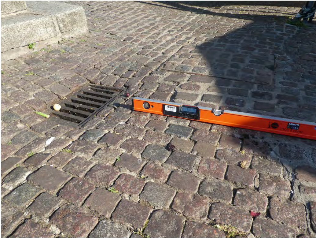
Photo 8: Zone 12 showing falls of 1 in 15 which is considered to be a ramp.
