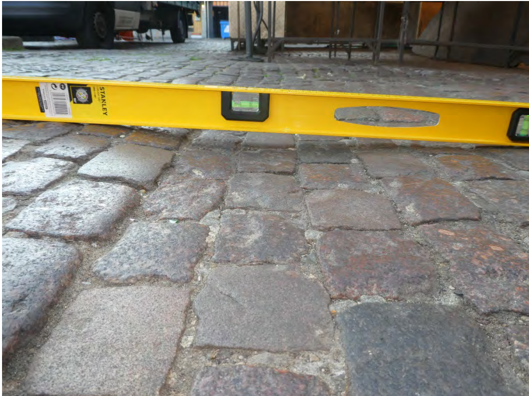
Photo 21: Undulation of 25mm on the edge of zone 3 and zone 11.
