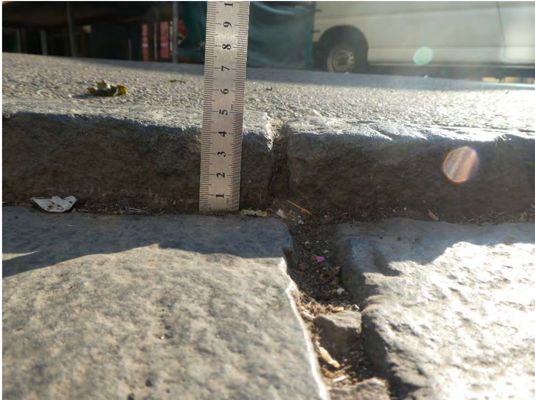
Photo 30: Lack of effective dropped kerb to south west corner.
