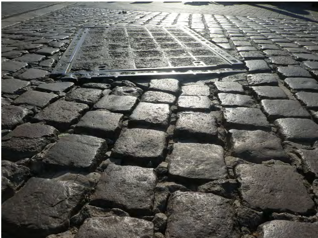
Photo 31: Missing pointing and uneven setts to north west crossing.
