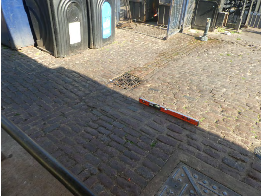
Photo 6: Surface in zone 11 with falls steep enough to be considered ramps.
