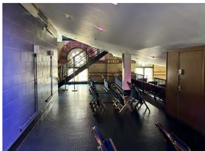
Audience members can bang their heads on the underside of the balcony - a major safety hazard. This zone feels claustrophobic.
