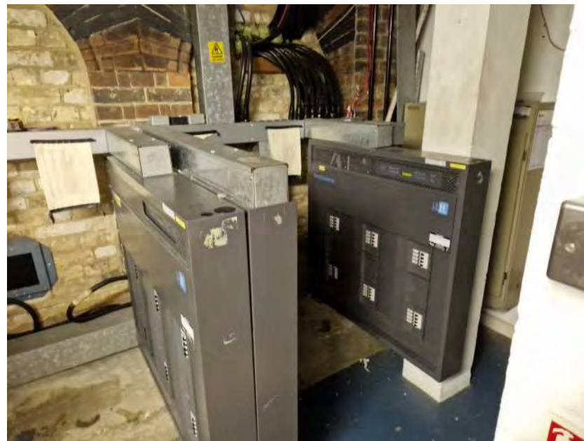
Existing Dimmer Location
