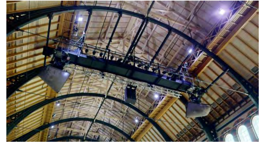
Existing Follow Spot Position
