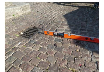
Photo 8: Zone 12 showing falls of 1 in 15 which is considered to be a ramp.
