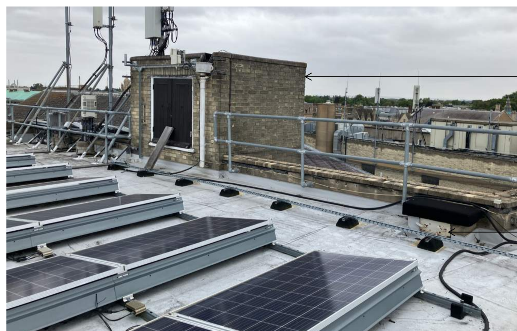
PHOTOGRAPH OF ROOF SHOWING PV, EDGE PROTECTION AND ACCESS BOX
