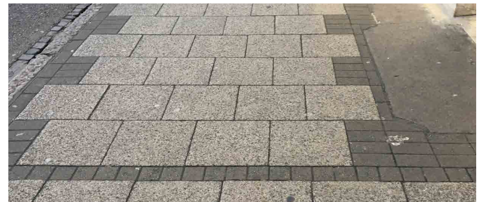
Bricks mixed with block paving
