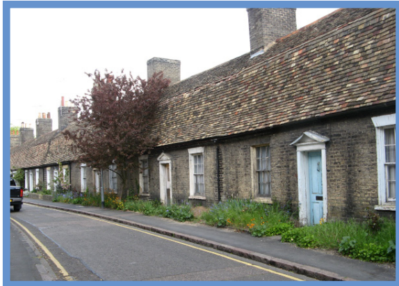
Nos. 7, 8 and 9 Orchard Street are suffering from neglect but have recently been sold
