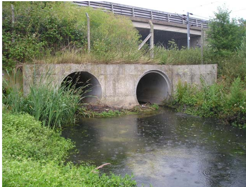
Figure B5.5: Triple Culverts under A14 (Smaller Culvert is Hidden by Vegetation on the Left Hand Side)
