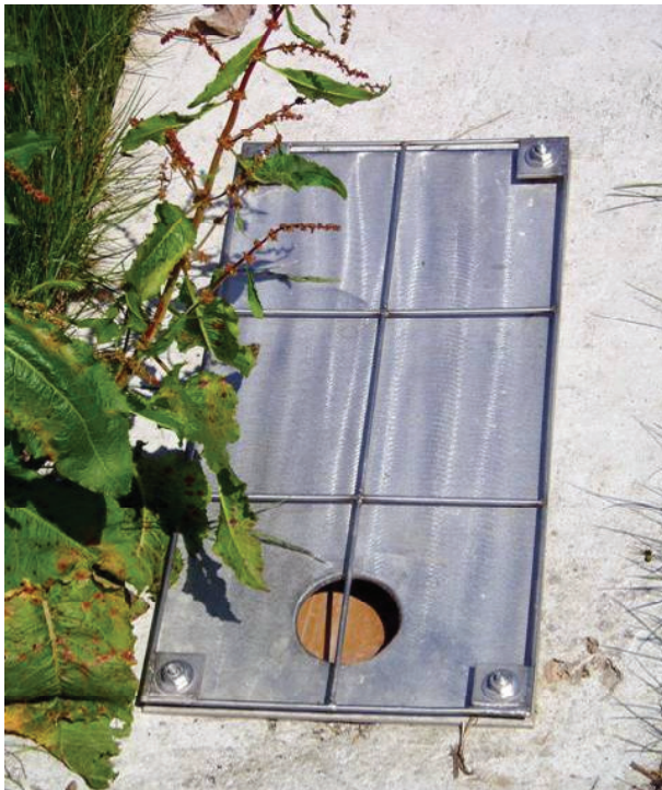
Orifice control to a basin located on the surface so that it is easily accessible
