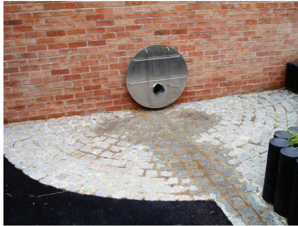
Stainless steel outlet leading to a surface rill
