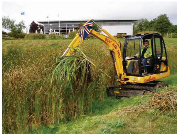
Managing wetland vegetation with a mini excavator. Larger excavators should not be necessary, motorway service area, M42
