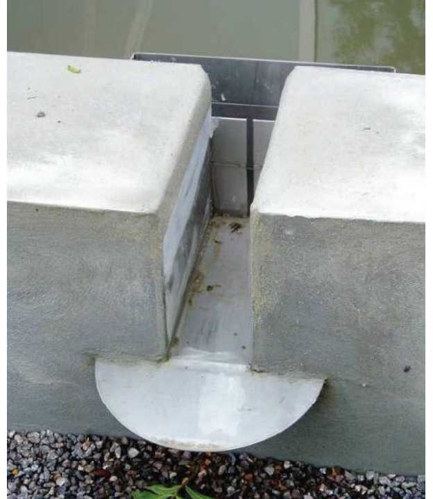
Slot weir outlet with steel plate to disperse water and debris guard behind
