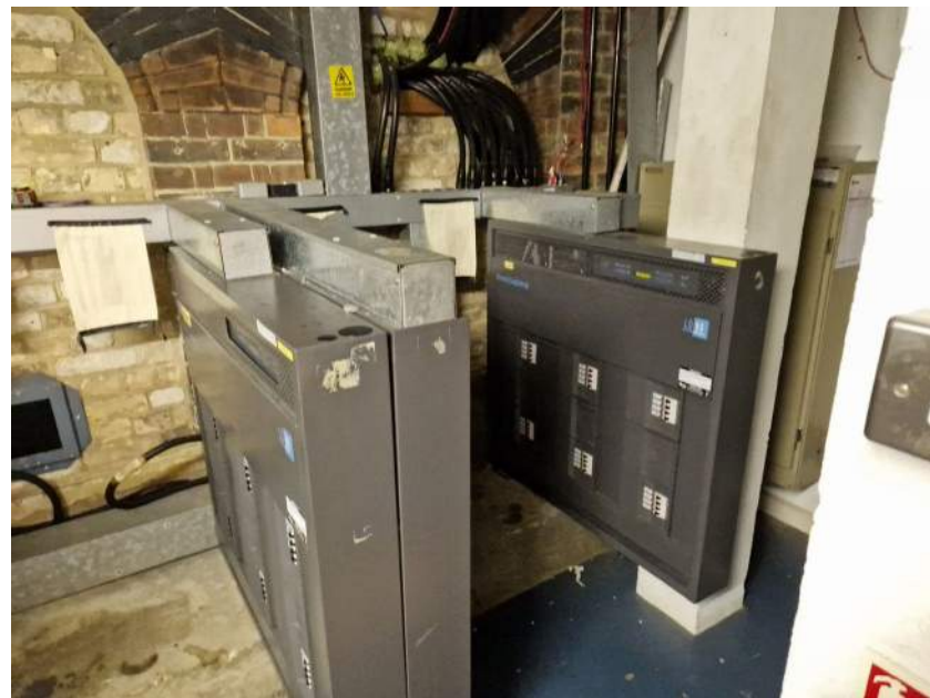
Existing Dimmer Location
