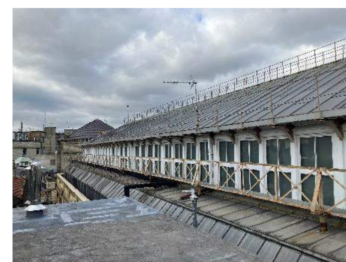
Clad auditorium supply plenum on west elevation forming thermal line.
