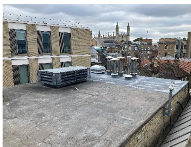
Flues and ventilation louvres above south plant room roof.
