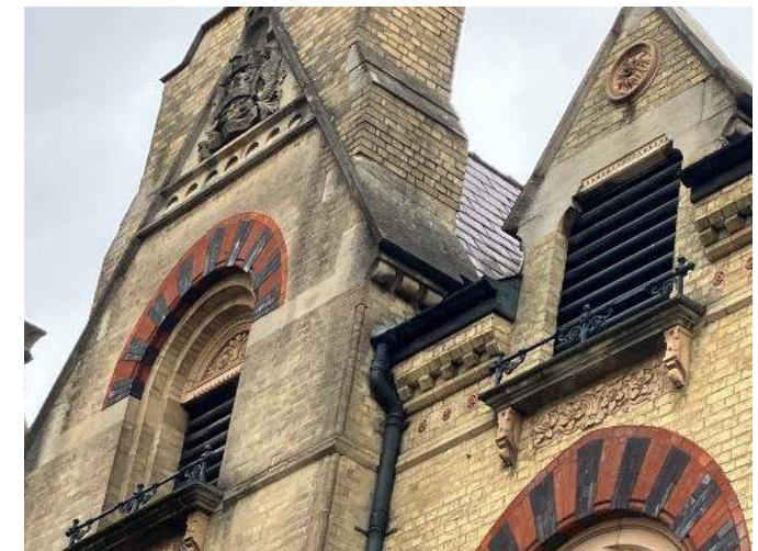
Flues and ventilation louvres above south plant room roof.
