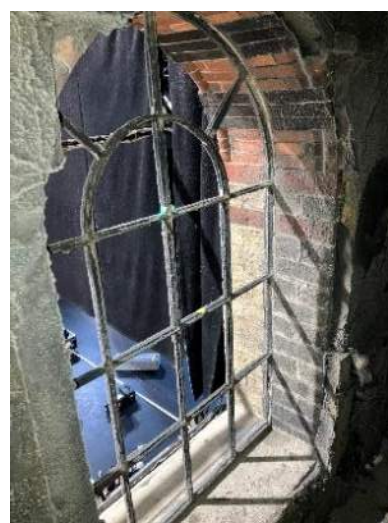
Auditorium return air path via window.
