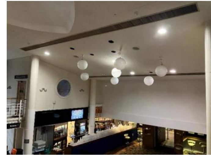
Ventilation grilles and lighting in foyer ceiling.
