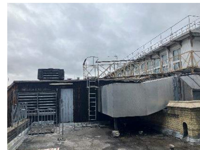
Supply duct from south plant room connects into auditorium supply plenum.
