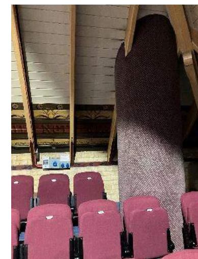
Foyer ventilation duct routing through auditorium balcony seating.
