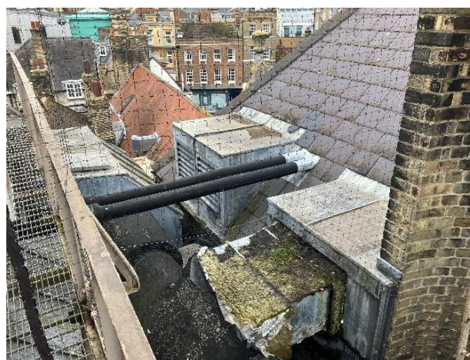
North plant room, supply duct leaving, splitting and setting into auditorium
