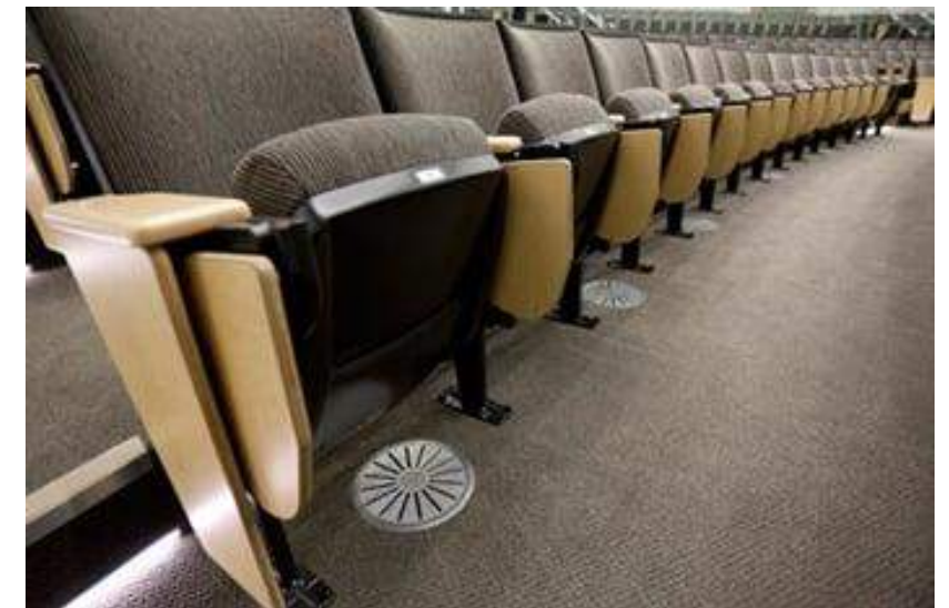
Typical in floor displacement ventilation terminals in auditoria
