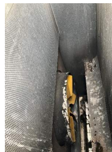
Typical smoke fan (external side).
