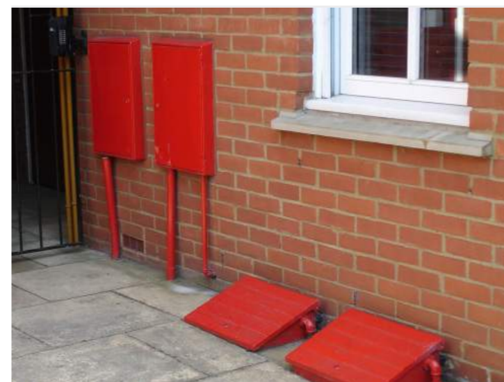
Avoid visual clutter from building services and service boxes
