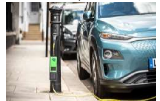
Dedicated street post charger
