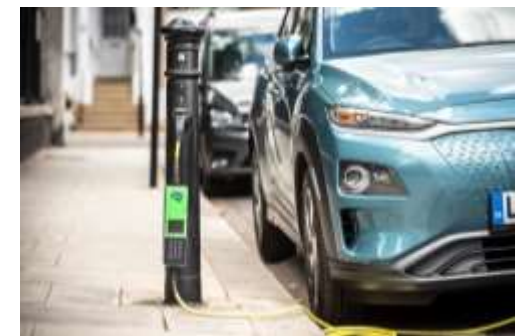
Dedicated street post charger
