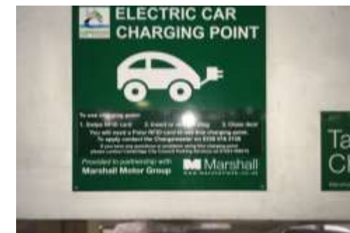
7kw charge point Queen Anne Terrace car park Cambridge
