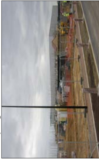
View looking south towards the Barrett Homes development from the central spine road
