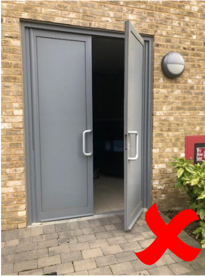
Fig 5 Double doors do not stay open and swing shut fast, hindering collections
