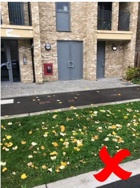
Fig 10 Swales mean there is no smooth access from bin store & bins have to be dragged across grass
