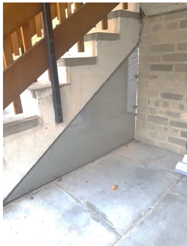
Perforated steel mesh under stairs for fire safety and cleaning at Rush Grove, Tenby, Cherry Hinton and many other blocks
