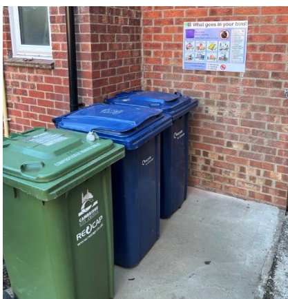
New hard standing under wheelie bins, with new signage to guide usage, at Ashbury & Golding
